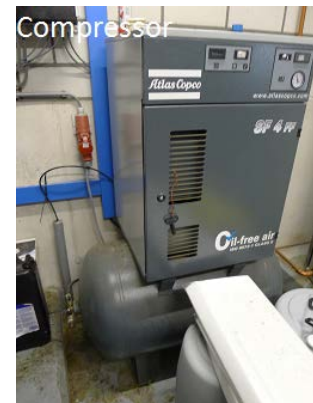
Figuur 7: Compressor (machinekamer)
