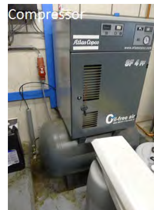
Figuur 7: Compressor (machinekamer)
