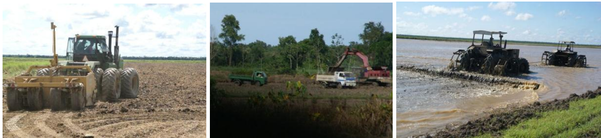
Figure 7 Levelling by scraper (left), hydraulic excavator (centre) both followed by puddling (right).
