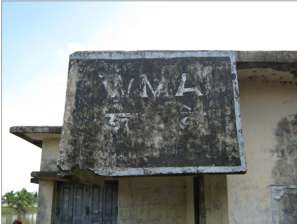
Figure 4.10. An abandoned WMA building in Arua, built during the KJDRP.
