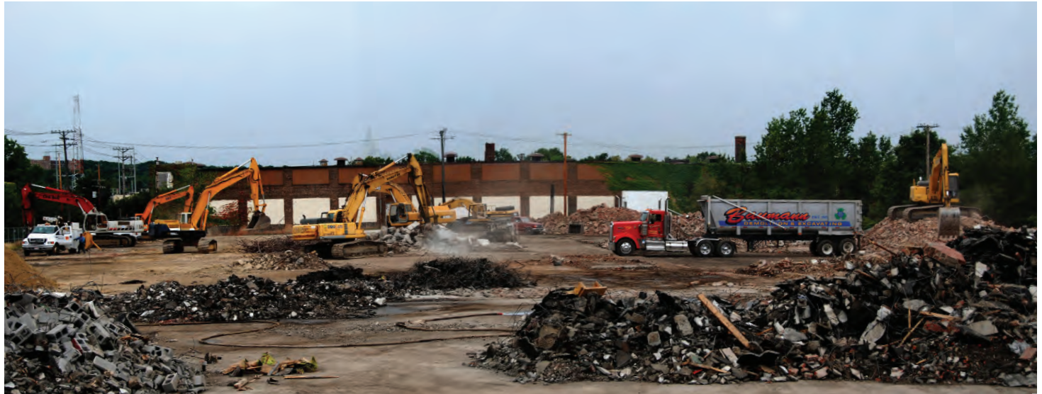
De-Zoning Demolition of GM's Fisher automotive body plant in Euclid, Ohio to make way for new expanding institutional campuses and business parks in the suburbs of Cleveland in the vicinity of Lake Erie. (Photo: ©2008 Pierre Bélanger)
