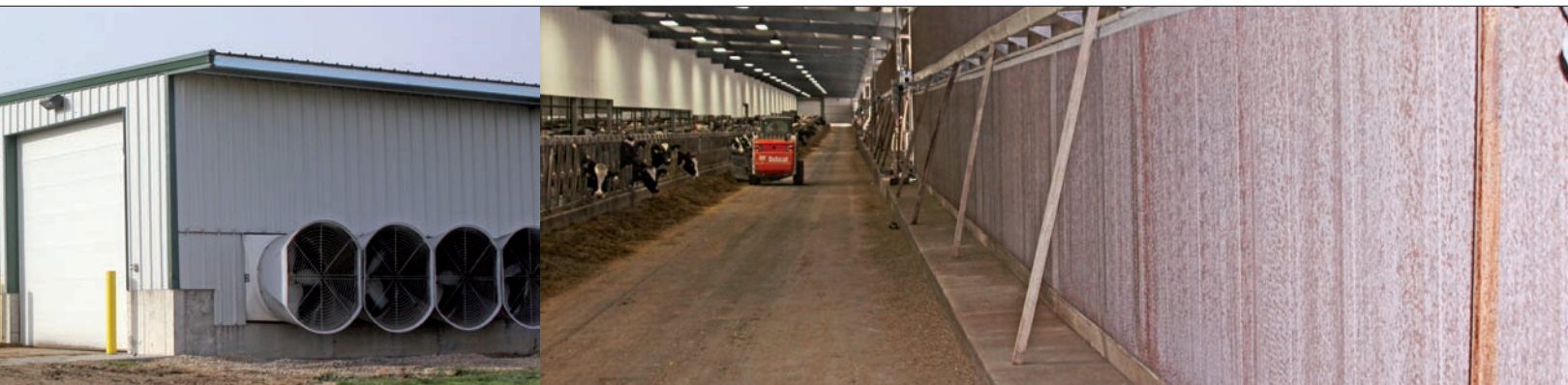
Climate control: air is water cooled by the cross ventilation system before entering the cow house
