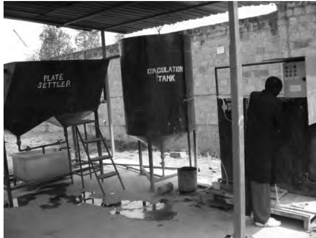
Photo Image 5-6 Part of the waste water treatment facility at Green Loop International (Photo by Leah Oyake-Ombis)
