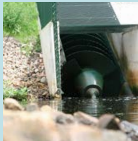
Archimedean turbine in The Netherlands (© Regional Water Authority Veluwe ).
