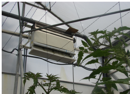
Fig. 2. Picture of one heat exchanger with the condensate water collection device.
