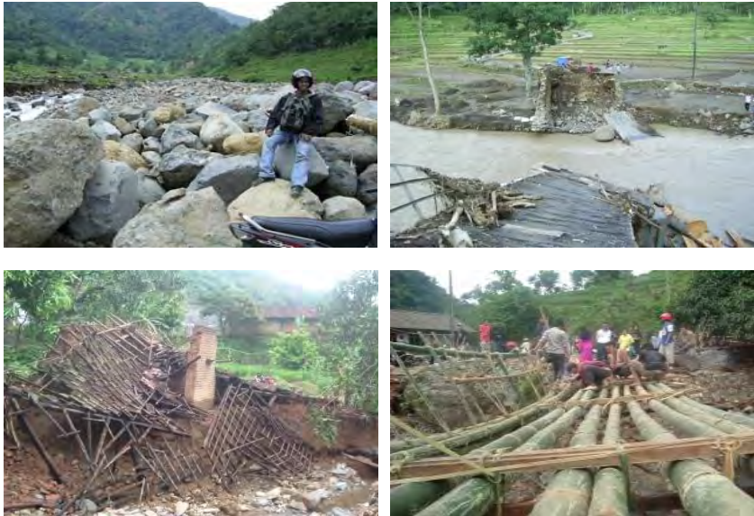
Figure 6.1 Damages after the flash flood in Tempur in 2006 and the construction of a temporary bridge (Makhali)
