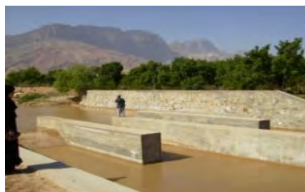
The intake fails to protect villages against floods
