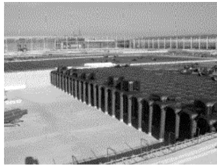
Fig. 1. Water storage under the greenhouse.
