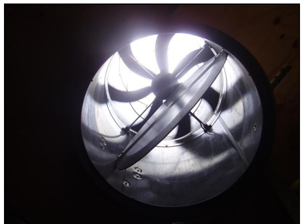
Detailfoto ventilator in schoorsteen zeecontainer
