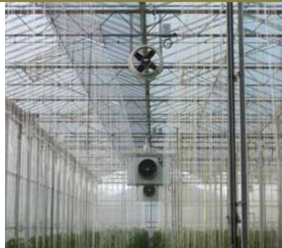
External air is warmed up, ensuring low relative humidity and drier crops
