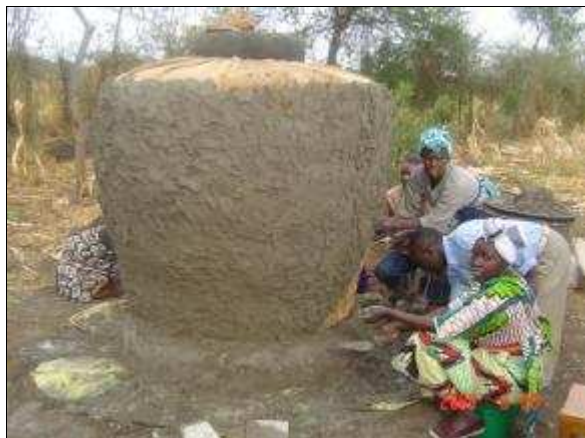
Water storage facility, for harvesting rain water
