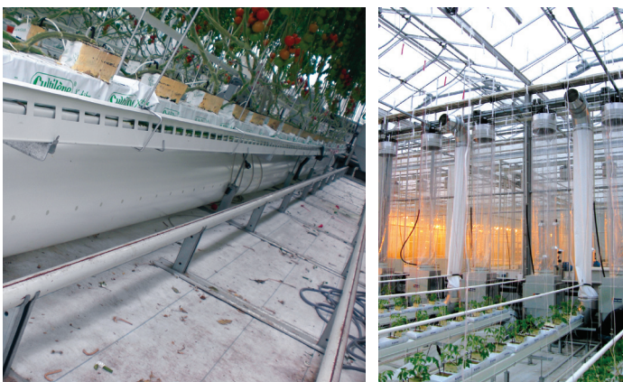
Figure 1. Blowing cool air into the greenhouse via horizontal ducts placed below the growing gutters (left picture), and blowing cool air into the top of the greenhouse via vertical ducts placed near the side walls (right picture).
