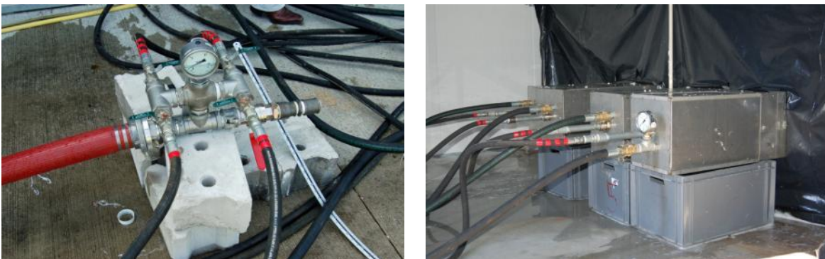
Figure 15 Pre-mix manifold and pressure gauge
