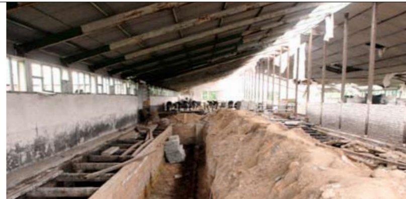
Dakplaten hingen los, overal lag puin
