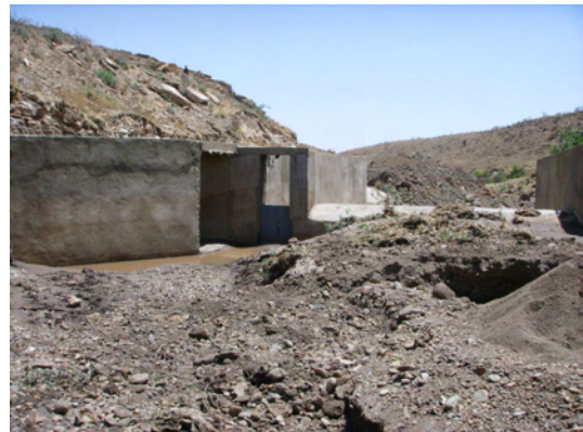
Figure 4.8: Sedimentation at the headworks
