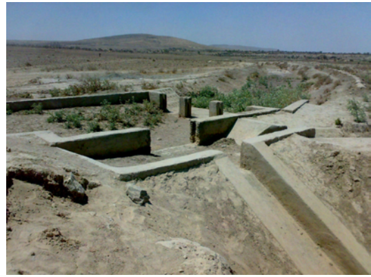
Figure 4.6: Division box at branch canal 5
