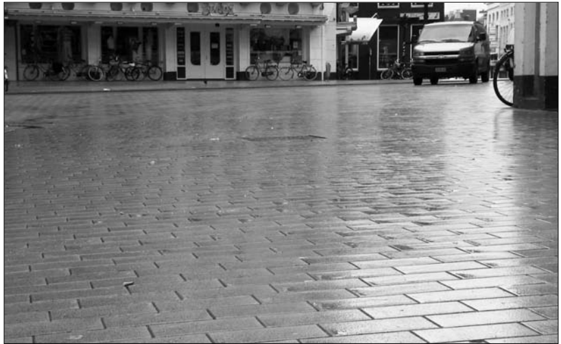
Fig. 3.14 Brightly coloured bricks à la Barcelona in Groningen's inner city, subjected to Dutch weather
