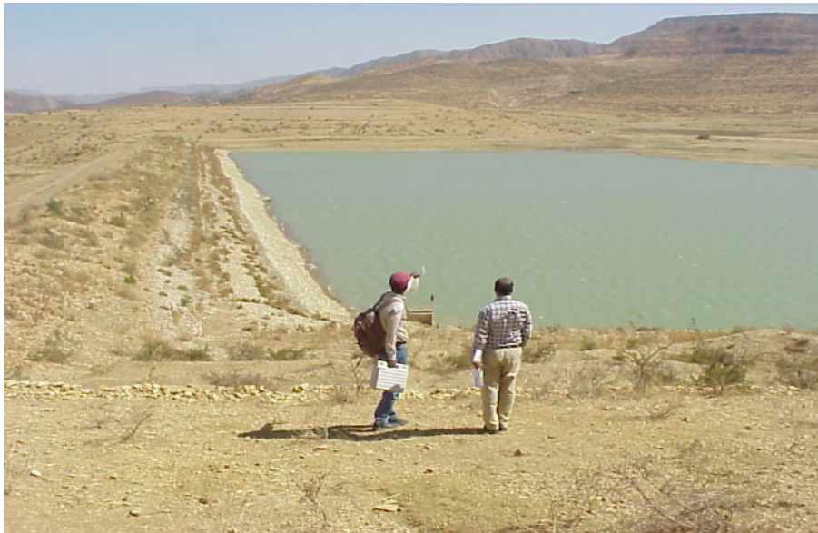
Figure 3.7 Partial view of the catchment area and the earthen dam at Korir irrigation scheme
