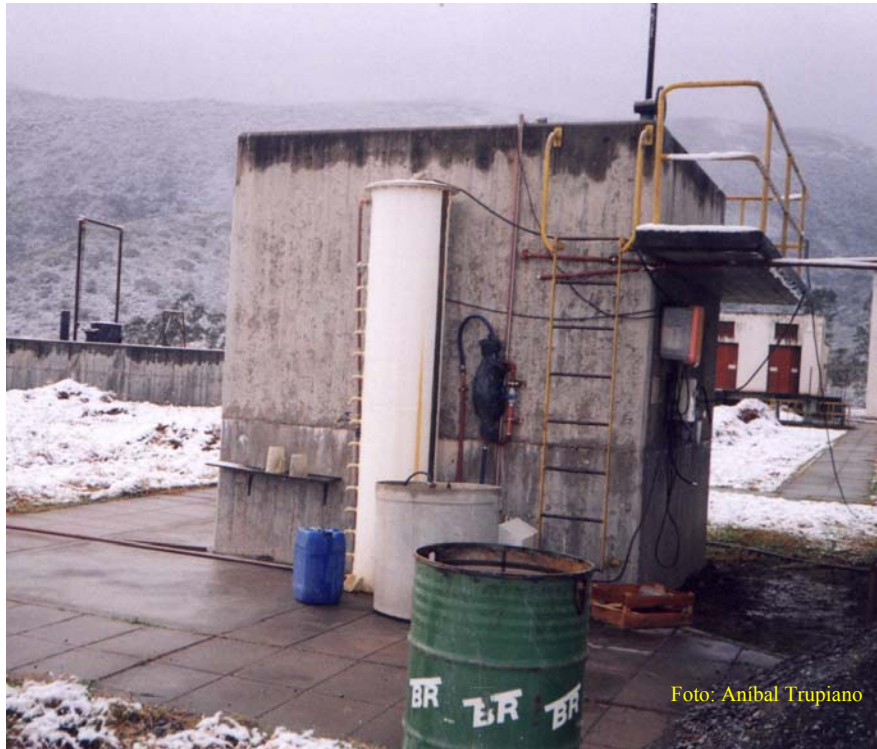
Figure 1. Pilot plant 1. Settler (not shown) and UASB reactor (white tank) on a background of “subtropical” snow.
