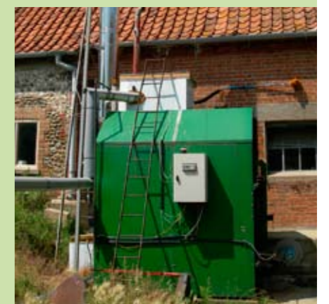
One of the existing energy generating burners at the Temple's unit
